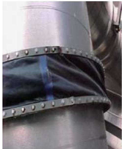
Large Duct Misalignment Causes Premature Failure
