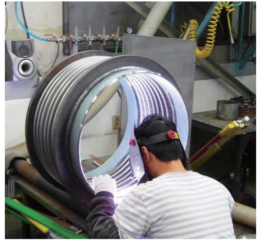
Kurbo's skilled welder using modern TIG welding for bellows and weld end attachment
