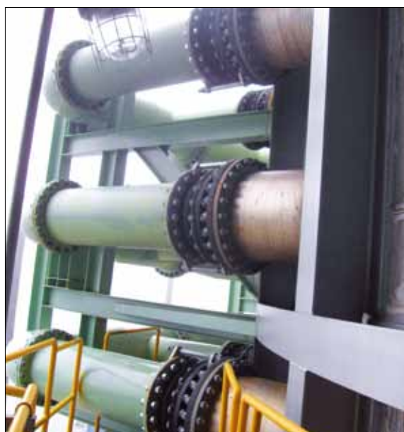
Type F21W-filled arch type joint in slurry line in thermal power plant.
