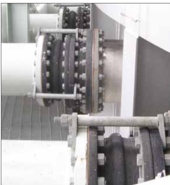
Viton expansion joints installation. Operating temperature about 180°C and flowing media of sulfuric acid.
