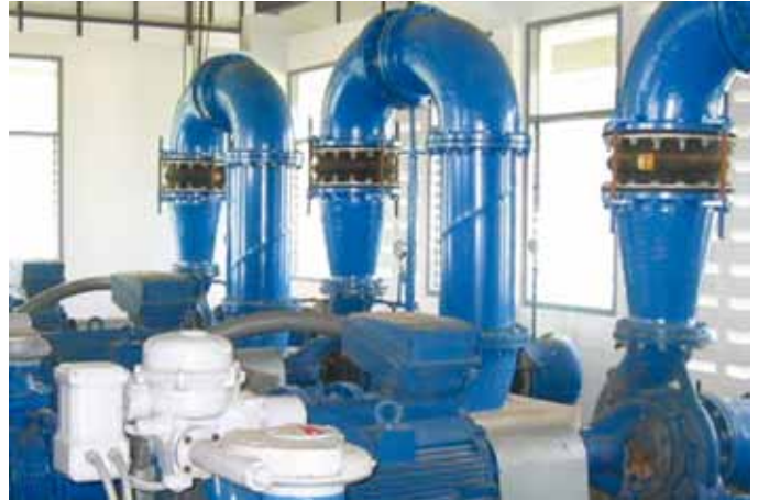
21W Expansion joints installed in suction and discharge connection at pumping station
